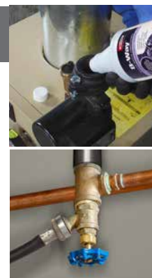
▲ Force pump drain line injection
