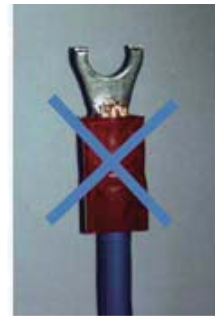
Terminal has been cut.
