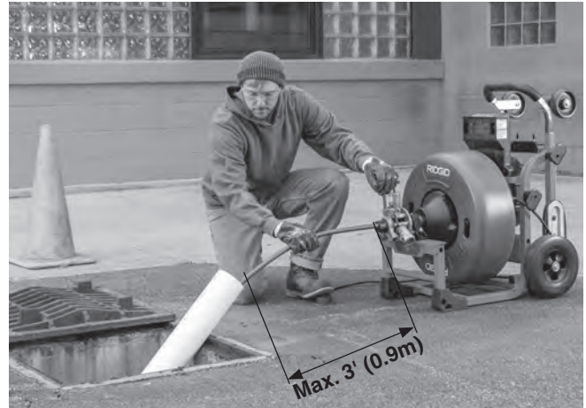
Figure 14 – Example of Extending Drain to within 3' of the Machine Cable Outlet
