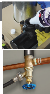
▲ Force pump drain line injection
