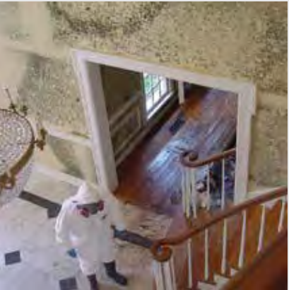
Water damage may lead to significant health concerns, lawsuits and costly insurance claims.
