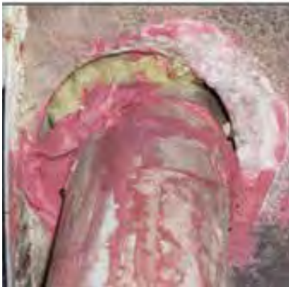
Commonly observed field-devised methods may provide a dangerous pathway for water, smoke, gas or fire.
